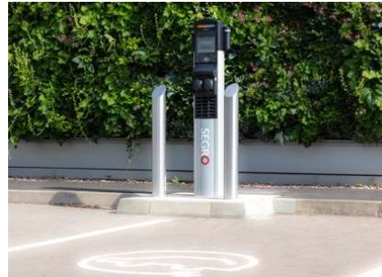
EV Charger (indicative)
